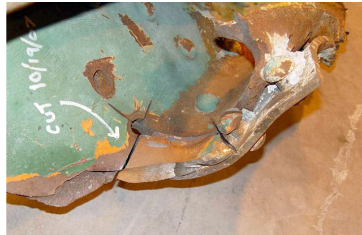
Fracture in a gusset plate
